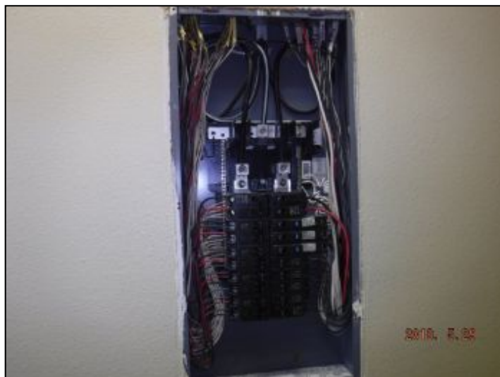
sub panel ok
