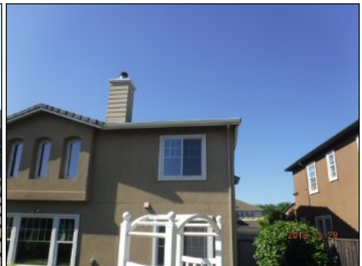
gutter slope poor
