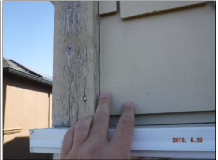
gaps at trim and siding
