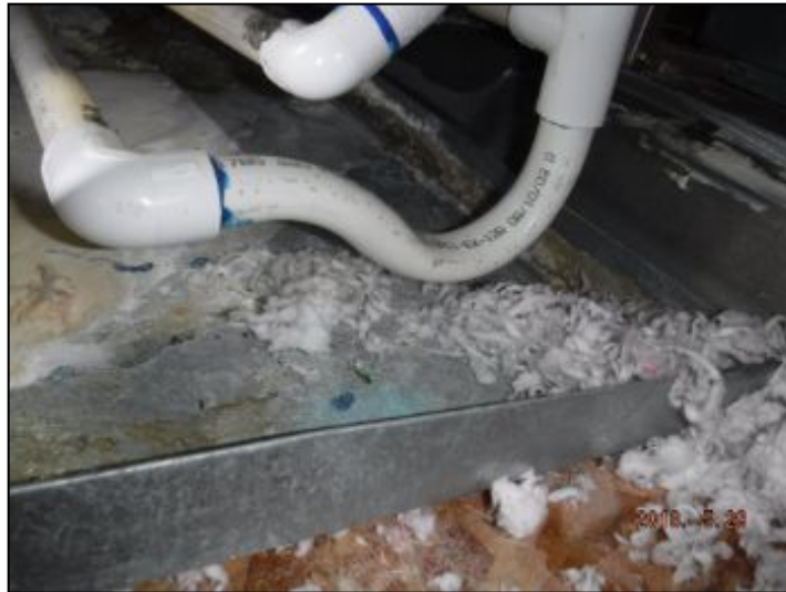
debris in pan
