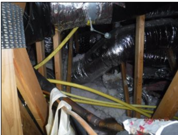
CSST gas lines
