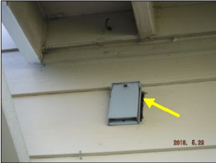
gaps at siding
