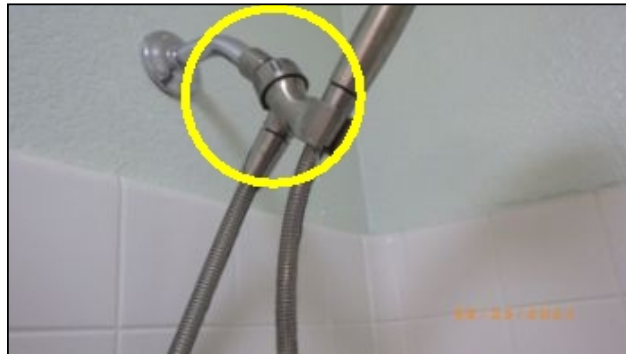
leaking shower head
