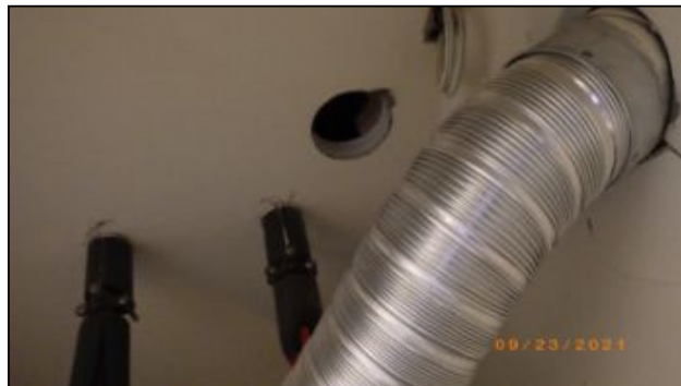
holes in firewall
