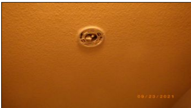
missing smoke detector
