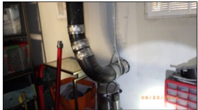
cast iron waste lines
