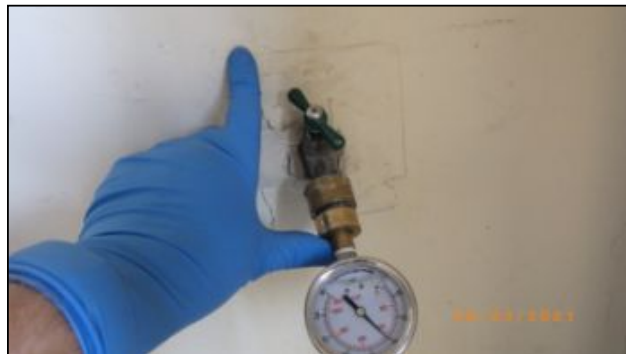
loose hose bib
