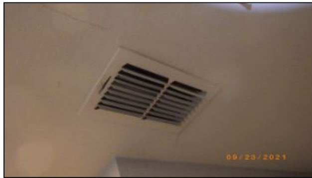
typical settlement cracks
